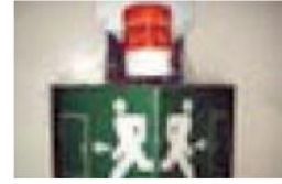
CTE – Strobe light mounted above door
