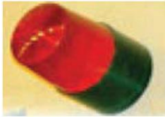
FCT/WVT - In an emergency, when you see flashing from the red coloured beacon lights mounted on the wall next to the service cabinets, leave the tunnel immediately
